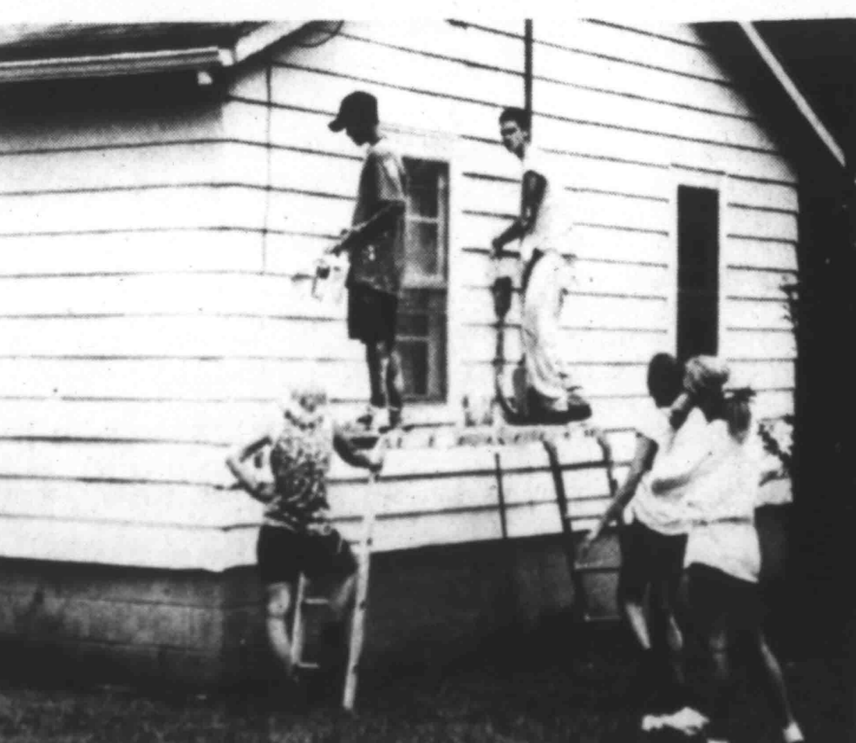
SARAH ROBERSON'S HOME at 9724 North 2nd Street in Gates is being painted.
