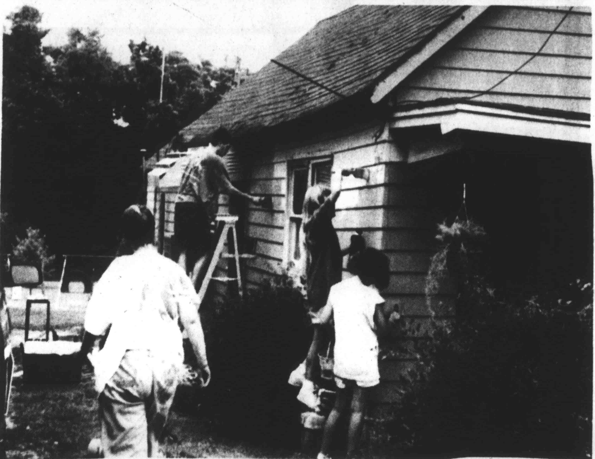
HELEN STRAYHORN'S HOME at 328 Huntington Street in Gates is being scraped and painted.
