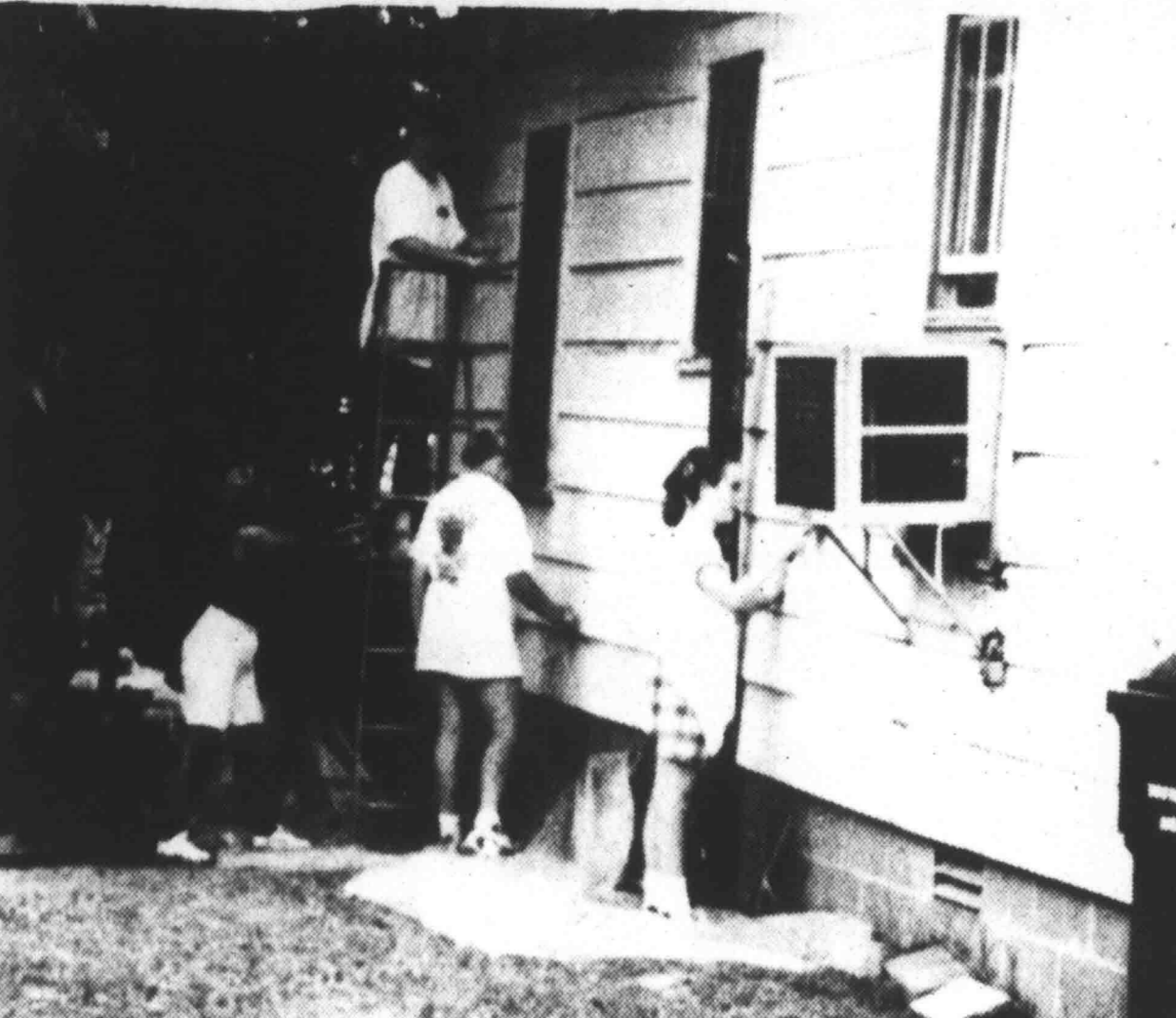
IVORY CLEVELAND'S HOME at 231 Pearl Street in Halls is being scraped in preparation for painting.
